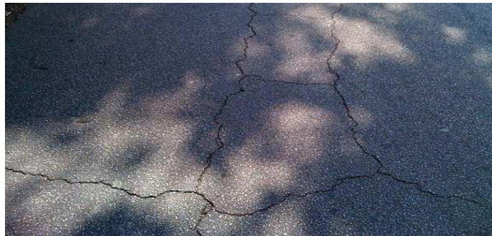
Gambar 2.5 Retak halus ( hair cracking )
