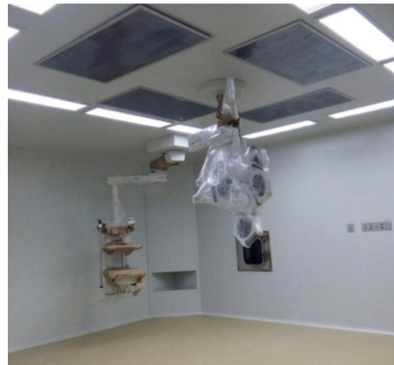
FIGURE 6. Hepa Filter Hospital.
