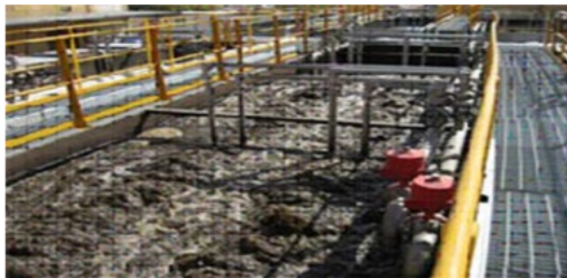
Gambar 9.5 Instalasi MBR Eden
