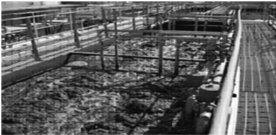
Gambar 6.4 Instalasi MBR Eden
