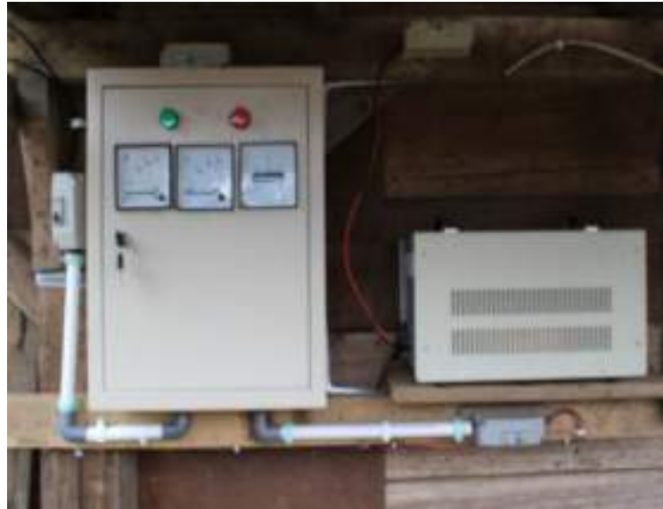
Gambar 31. Panel kontrol ELC ( Electronic Load Controller )
