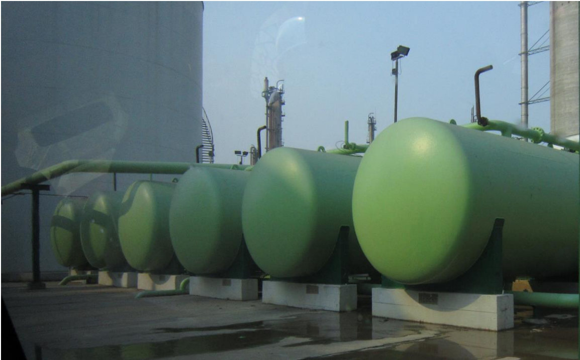
Gambar.... Back Wash Sandfilter
