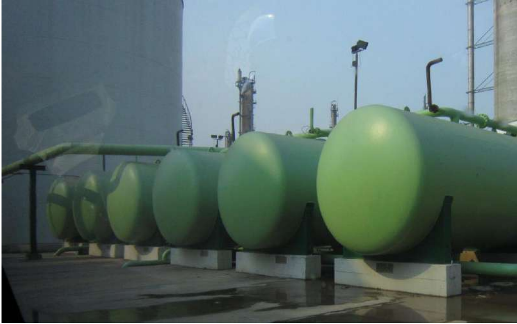
Gambar 11.. Back Wash Sandfilter
